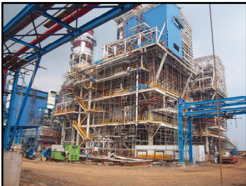
Figure1. Heat recovery steam generator (HRSG) of Tanjung priok gas fired power plant extension project under construction.
