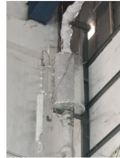
Gambar 5. Water Cooling Tank
