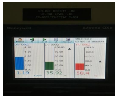
Gambar 2. Kontrol Panel Volume Tangki
