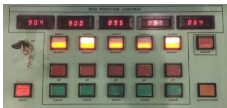
Gambar 5. Panel kontrol batang kendali reaktor
