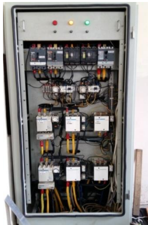
Gambar 13. Panel pompa pending sekunder.
